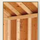
Double 2" x 4" top plate on all side walls over 18' long and A-Frames over 16' long.
